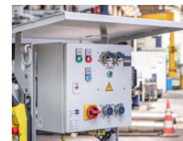
Key-operated solenoid-controlled HST-M in a customised enclosure
